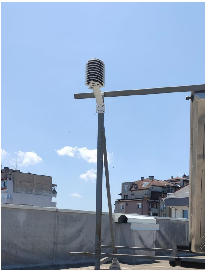
Figure 14 The Barani Design weather station installed at the OP32 Burgas Observer Project © EnEffect
