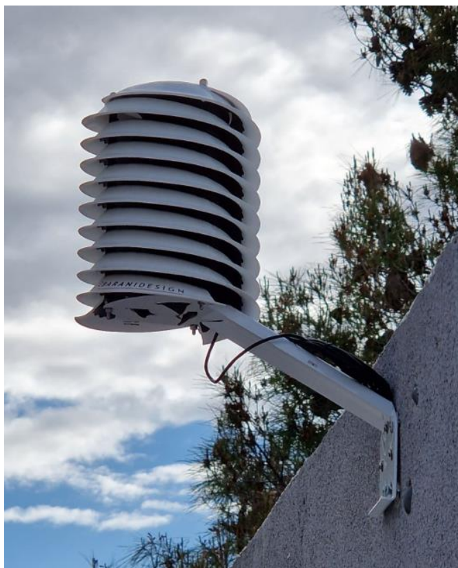
Figure 2 The weather station installed in case study 2 ©Hellenic Passive House Institute
