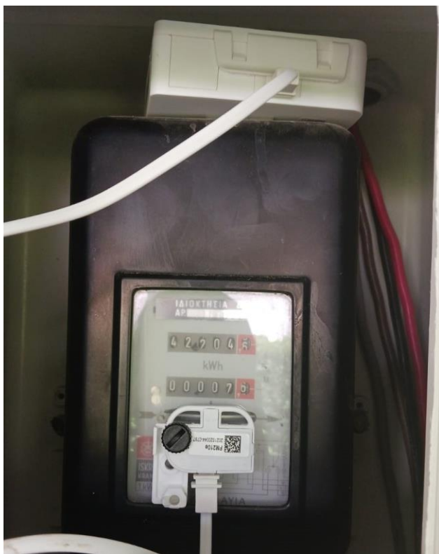
Figure 8 The Fludia energy meter being installed on case study 2 ©Hellenic Passive House Institute
