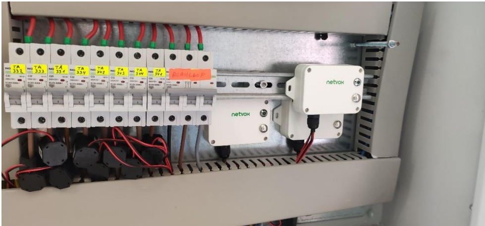
Figure 13 The Netvox energy meters installed at the OP32 Burgas Observer Project © EnEffect
