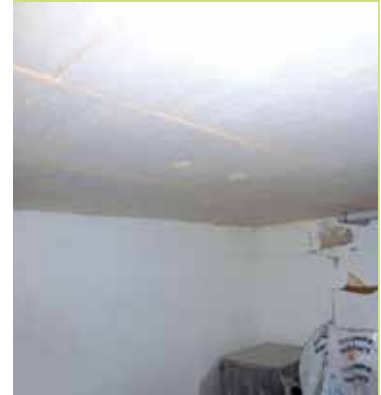
Photo: Basement ceiling insulation with dowels – additional mechanical fixing using dowels ensures the basement ceiling insulation is kept in place.
