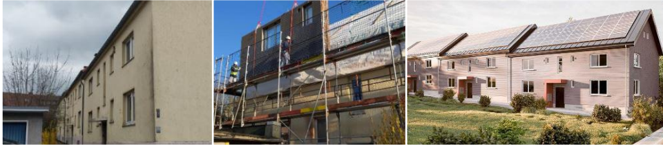
Serial retrofit of residential buildings built in the 1930s in Hameln (Germany) using prefabricated elements. The installation of an insulation element just took 20 minutes. © ecoworks
