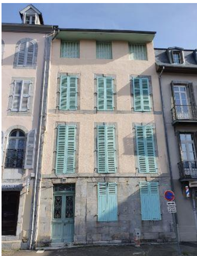
Retrofitting is urgently needed for this apartment block in Bagnères de Bigorre in the French Pyrenees. © F. Colas
