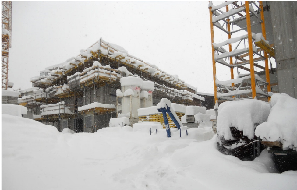
Photo of typical winter conditions in Sankt Johann in Tirol at the construction site of ST16-17; ©NHT
