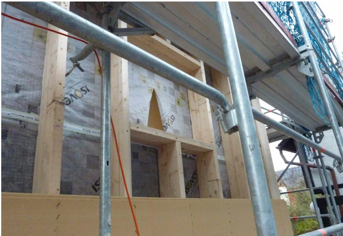
Stud wall façade with wood fiber boards before cellulose filling. Windows to be installed later into these wooden beam frames. Source: PHI
